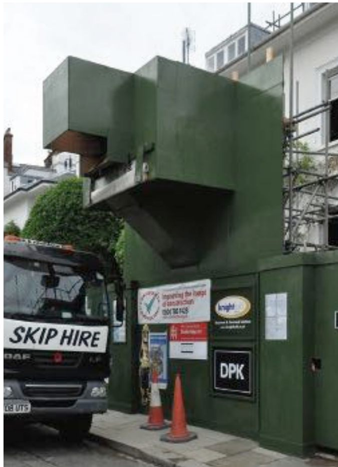
3-4 Albert Place basement work without suspension of parking place for the skip
